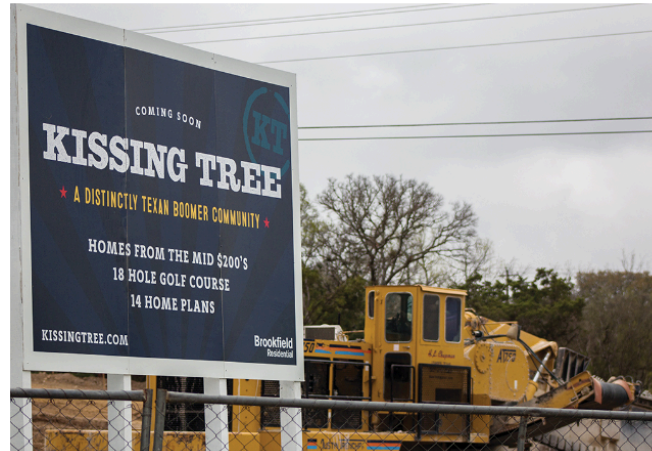
Photo by: Pablo Mejia | Staff Photographer Construction site for Kissing Tree community March 4.
